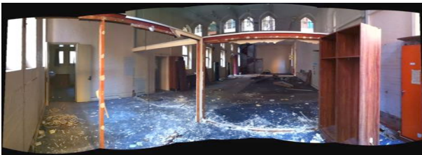
A 180° view of the 'gutted' Sussex St interior – taken from the remains of the PC's Office.
