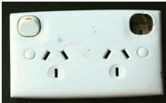
A loose switch to a power point needs repair as soon as possible
