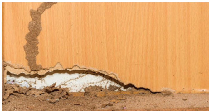
These mud deposits indicate active termites
