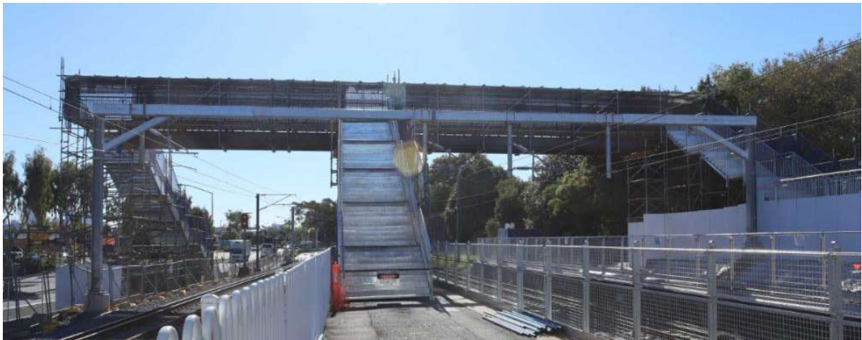
Image – A view of the temporary scaffold pedestrian overpass from Yeronga station.
