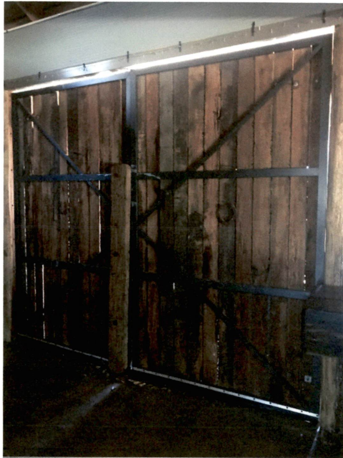
FIGURE 2 – AIR GAPS REQUIRING NOISE CONTROL
