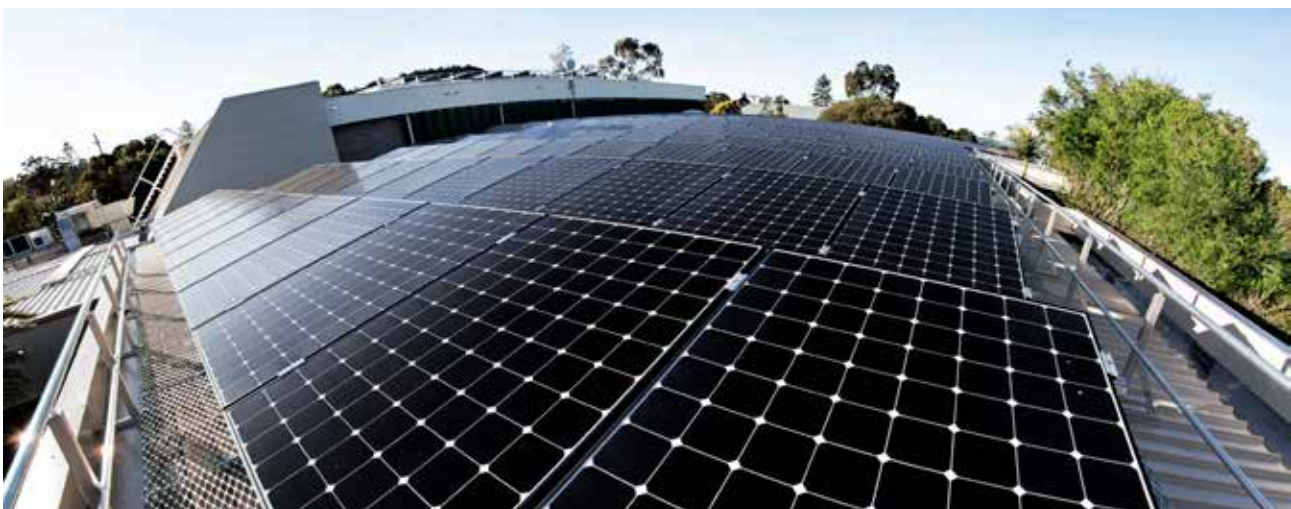
Lake Macquarie City Administrative Centre solar panels.
