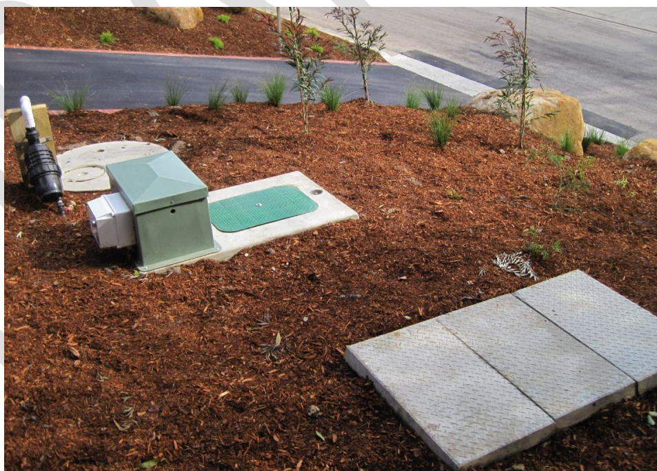
Figure 2: Treatment Plant with sub-surface irrigation
