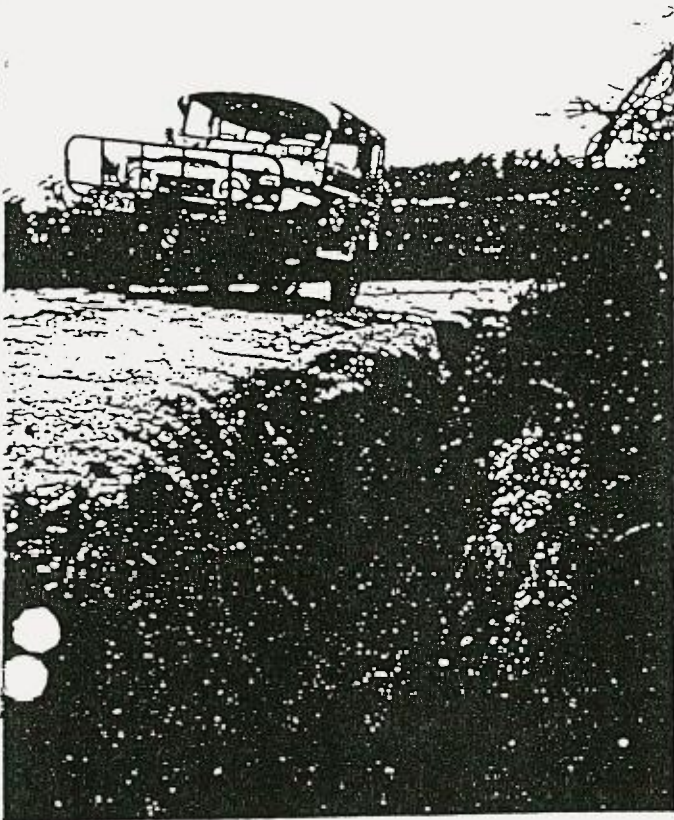
Figure 5 Gullying of table drains is a serious erosion problem and a danger to road users.
