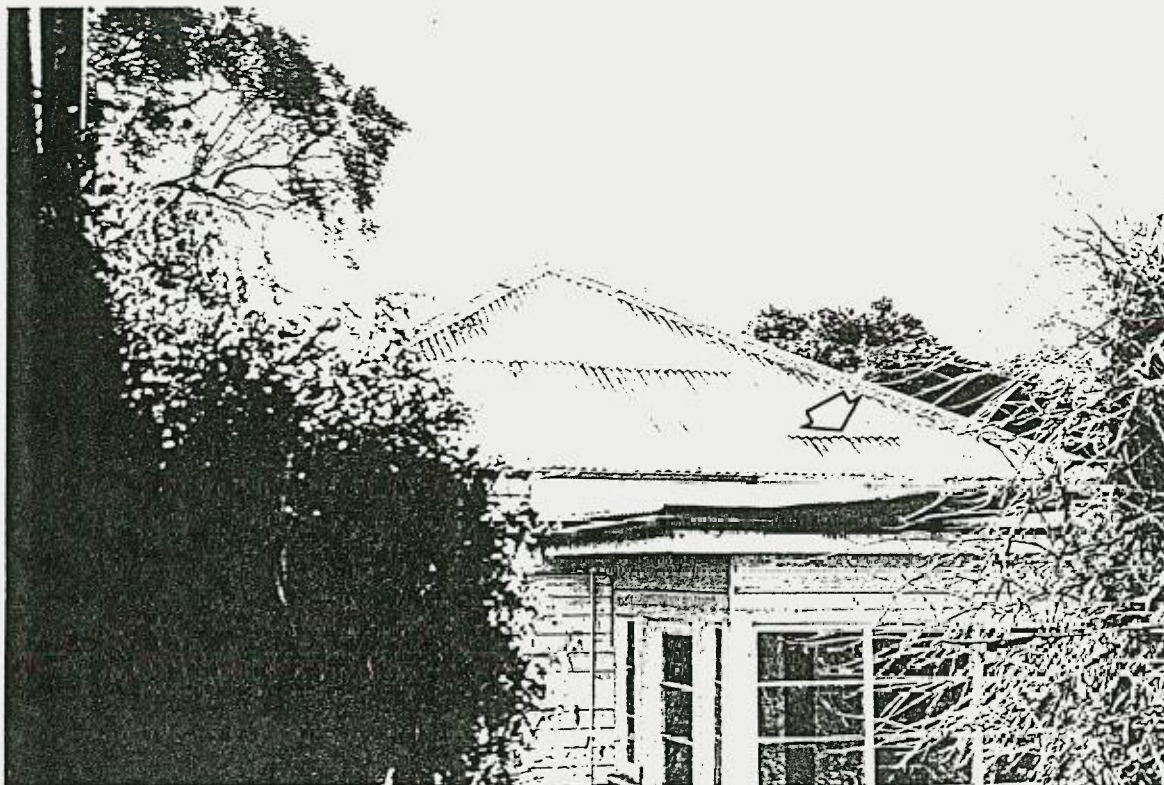
Photo 4. Detail of southern hip of main roof, "Minnaville" homestead. Location of former chimney within main roof line is shown by roofing sheets (arrowed).
