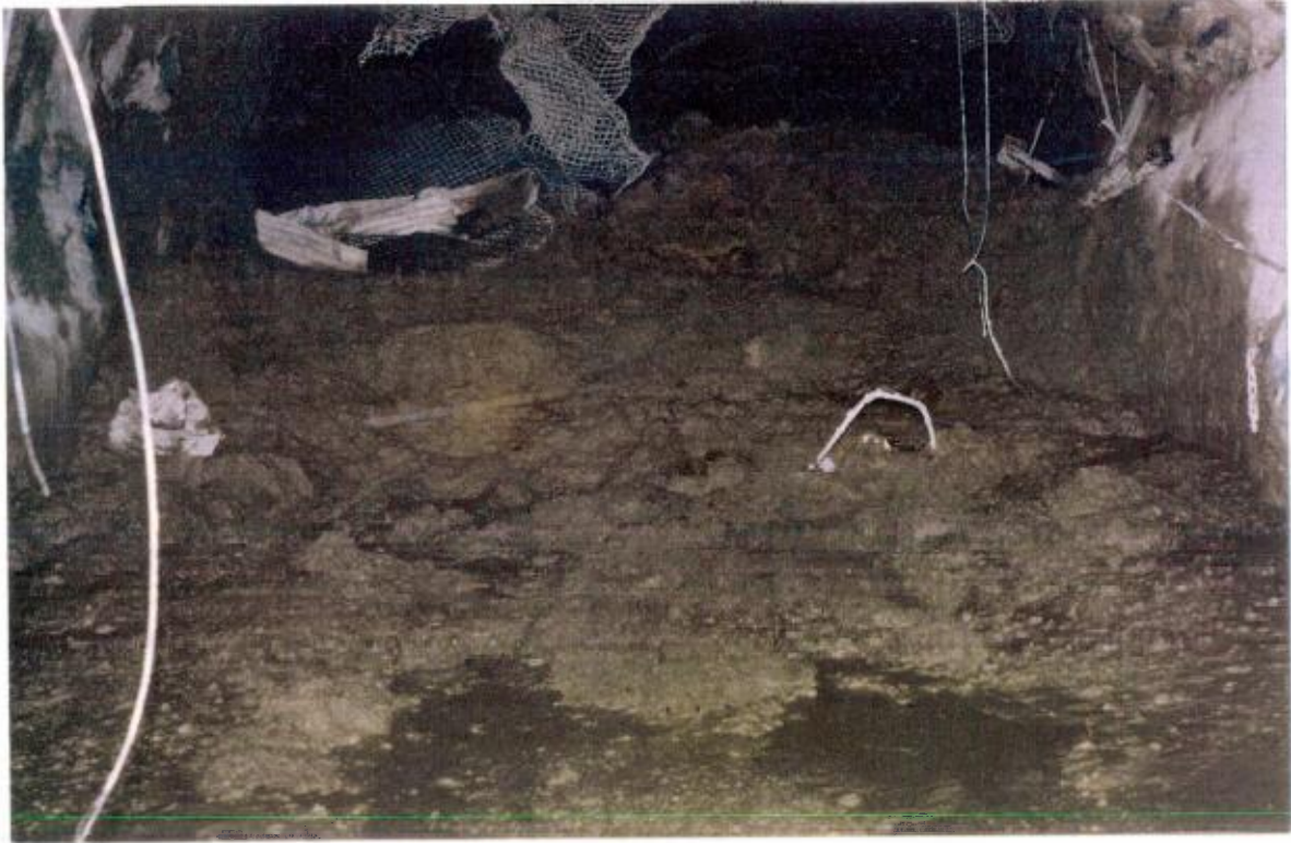
18 March 1996 3 Haulage EPD North of Fuel Store Showing fill flow Consistency of fill - Foreground - Sloppy - Rear - Firm and putty like
