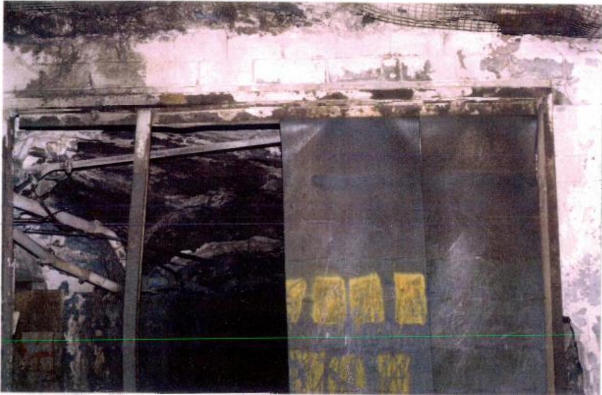
18 March 1996 2H Plat Area Undamaged vent curtain
