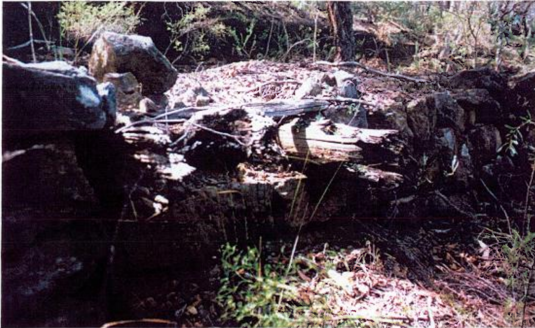
Timber Culvert, near Mitchell's Loop, Dharug NP (Section 3). Collapsed, rotted, burnt and silted up, causing structural failure.
