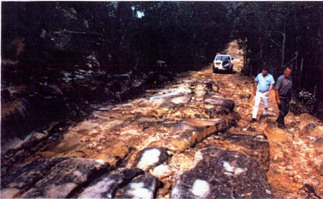
Eroded road section. All original pavement lost, road levels eroded by 0.5 to 1 metre. Photograph taken 6 km north of Wisemans Ferry in Dharug NP (Section 3).
