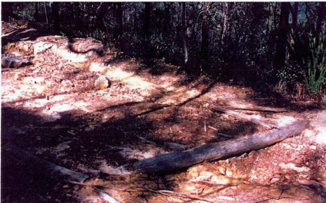
Timber Culvert, near Mitchell's Loop, Dharug NP (Section 3). Erosion of road overburden has exposed top slabs and beams, causing collapse.
