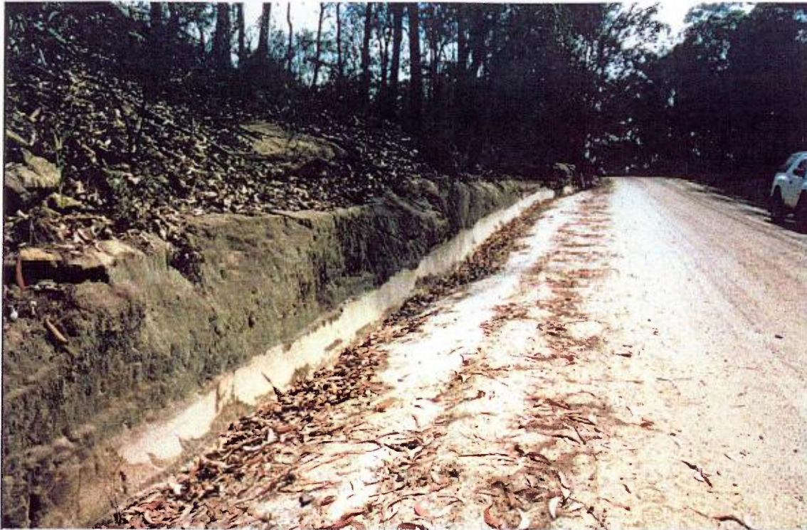
Long section of damaged side cutting, south side of road.
