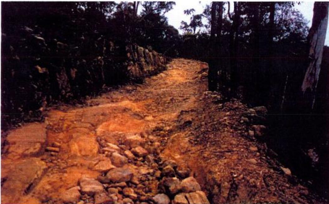
Eroded road section. Original pavement level on right. Foreground eroded by 1 metre. Photograph taken near Sampsons Pass adjacent to Yengo NP (Section 3).
