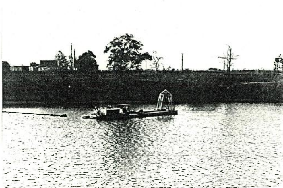
PLATE 16: Sand dredge with floating pipeline on Hawkesbury River, Windsor (Monier Pty. Ltd.).
