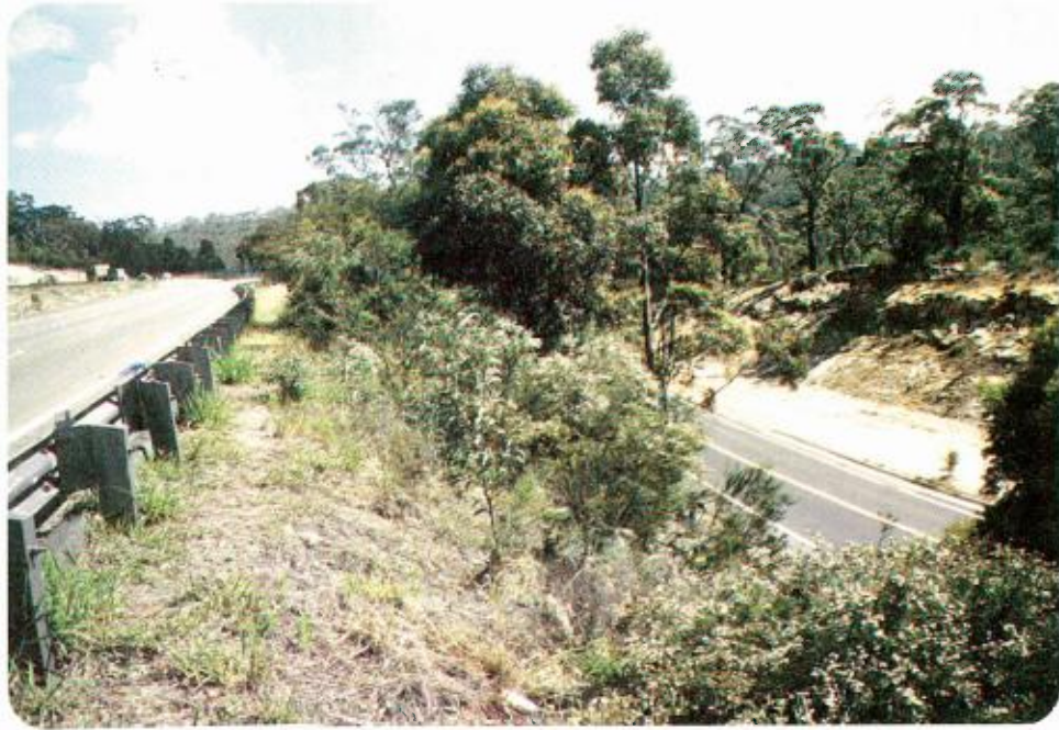
(13) Regeneration on Sydney-Newcastle Freeway (SECTION 9.2.8)
