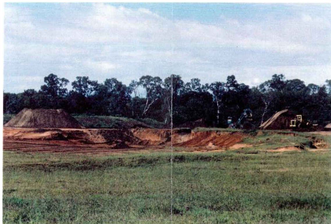
FIGURE 13 - Sand Extraction Area and Riverside Soil Processing and Stockpiles on Eastern Side of Property
