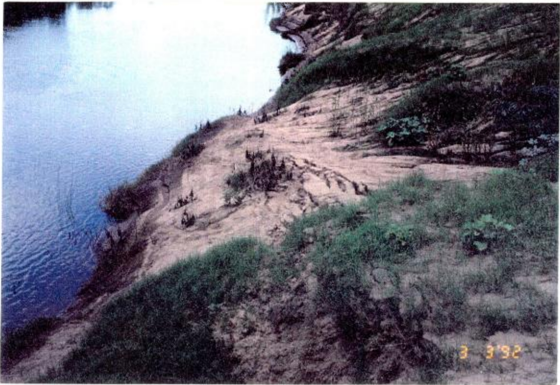
FIGURE 33 - Scouring and Tension Cracks in River Bank of Spring Farm at Eastern End of "Knoll" area
