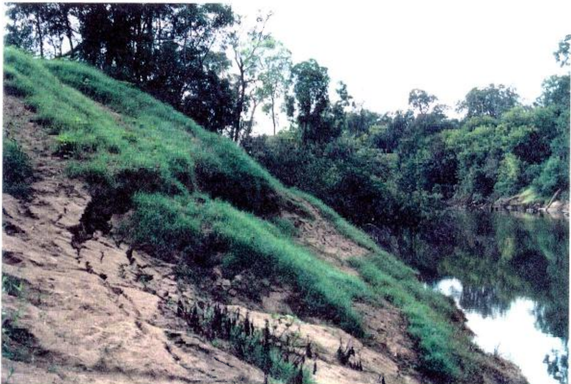
FIGURE 34 - Tension Cracks and Slumping in North Bank of Nepean River in Area with High Soil Bank
