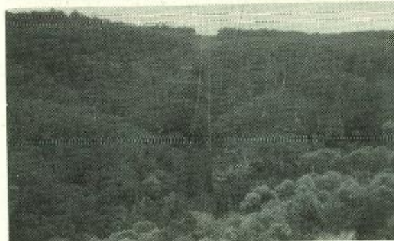
ZONE 3 SINGLE TRANSMISSION LINE OVER KATOOMBA CREEK The eastern 66kV transmission line crosses Katoomba Creek in a gully span parallel to the 132kV line, on the left side of the photograph.
