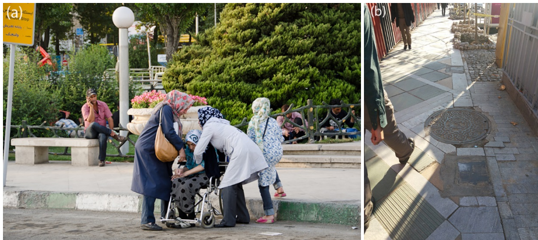
Figure 8. (a) Difficulty for using the street for people with disabilities due to uneven surfaces and absence of kerb ramp. Tadjrish square (Photo by Kamyar Adl- Flickr user); (b) gradual destruction of pavements due to improper implementation and lack of maintenance caused difficulty for pedestrians (Photo by Roya Salimzadeh).
