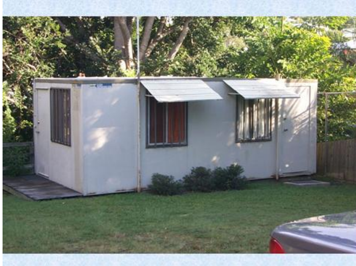
This was the church office, photocopy room and storeroom. It was infested with ants, it was hot and it leaked so bad.
