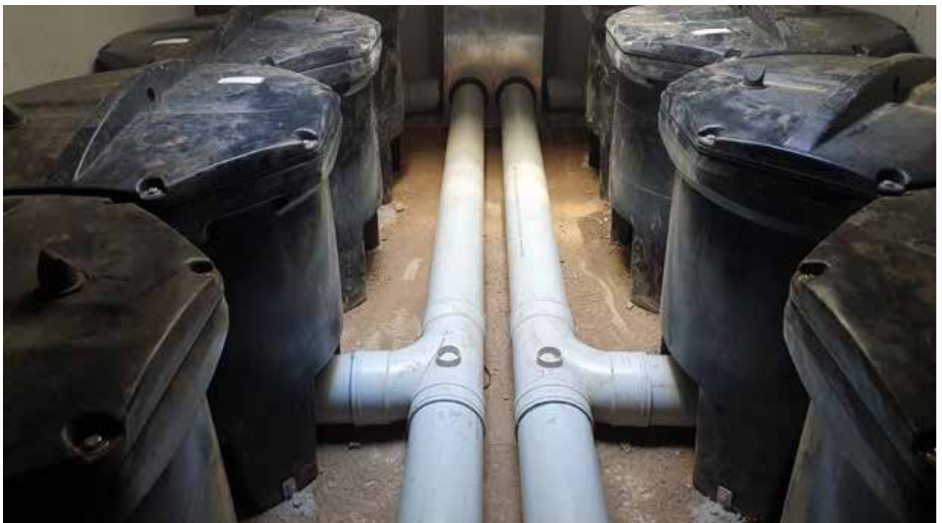
Figure 1 - SPELFilters in a concrete chamber / vault
