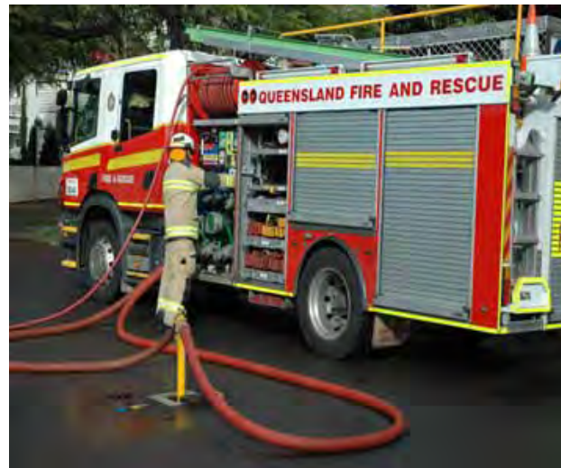
Figure 2 – Use of Hydrant System
