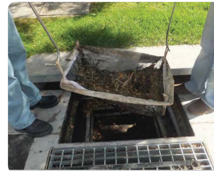
Photo 14 Lift the bag from the stormwater pit
