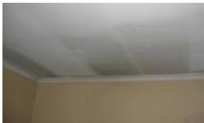
Figure 2: Mould growth causes staining on a ceiling.
