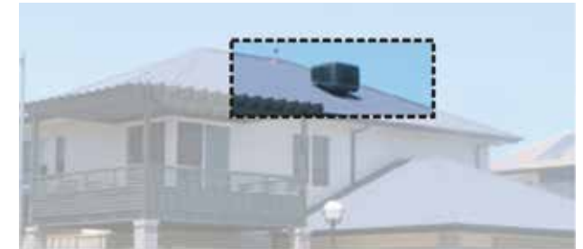
Figure 40. Air conditioning or service related equipment must not be visible from public view
