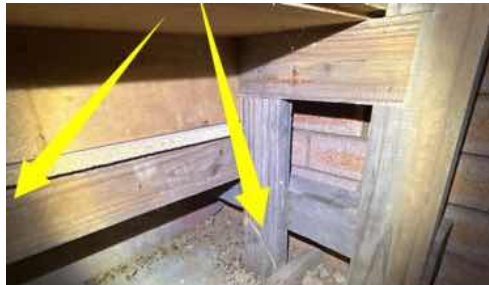
Example of termite workings in stairs adjacent to the bathroom
