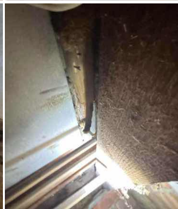
Example of termite workings in sole plates, photo from beneath the bathroom
