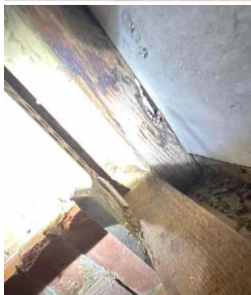
Example of termite workings in joists and sole plates, photo from beneath the bathroom
