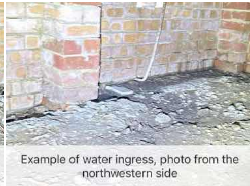
Example of water ingress, photo from the northwestern side
