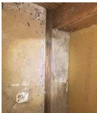
Example of termite workings in top plates, photo from above the bathroom
