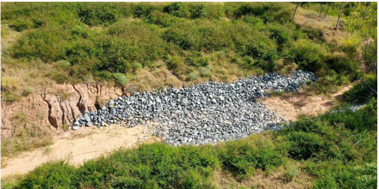
Figure 10 Rock Chute 4 looking south, evidence of rill and gully erosion on batter. photo supplied by Verterra.
