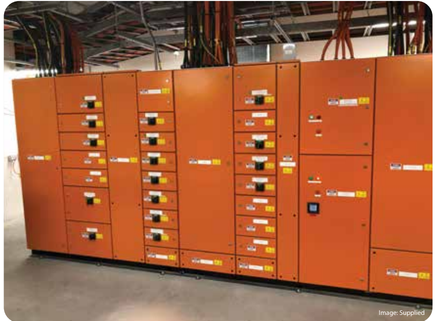
Fuji SMBE Macquarie supplied hundreds of switchboards with customised functions to Star Electrical, the lead contractor for the John Hunter Health and Innovation Precinct.
