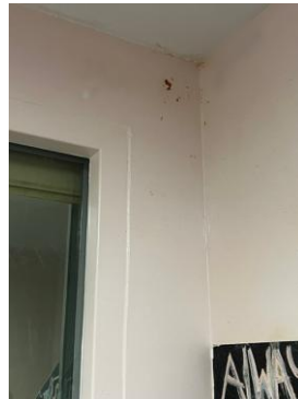
Image 21: Food and stains on wall in bedroom
