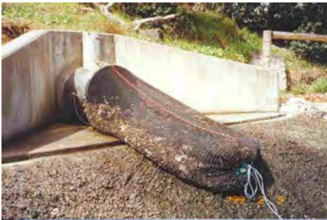
Photo: Gross pollutant trap at Umina, Gosford City Council, New South Wales (Source: www.gosford.nsw.gov.au ).
