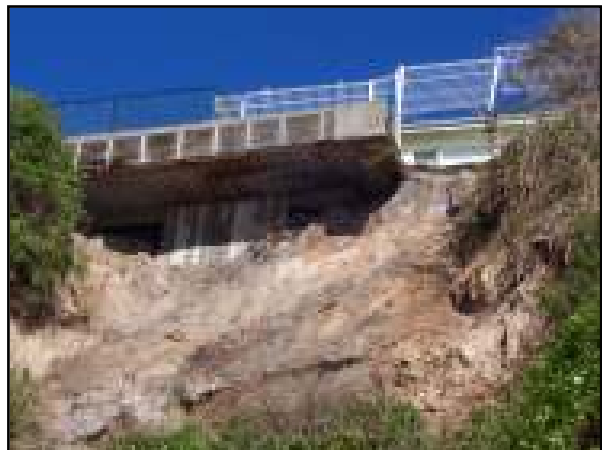
Figure 6d: Landslide at Cabbage Tree Harbour, Norah Head exposing overhanging deck structure on 22 nd June 2007 (Courtesy Department Environment & Climate Change)
