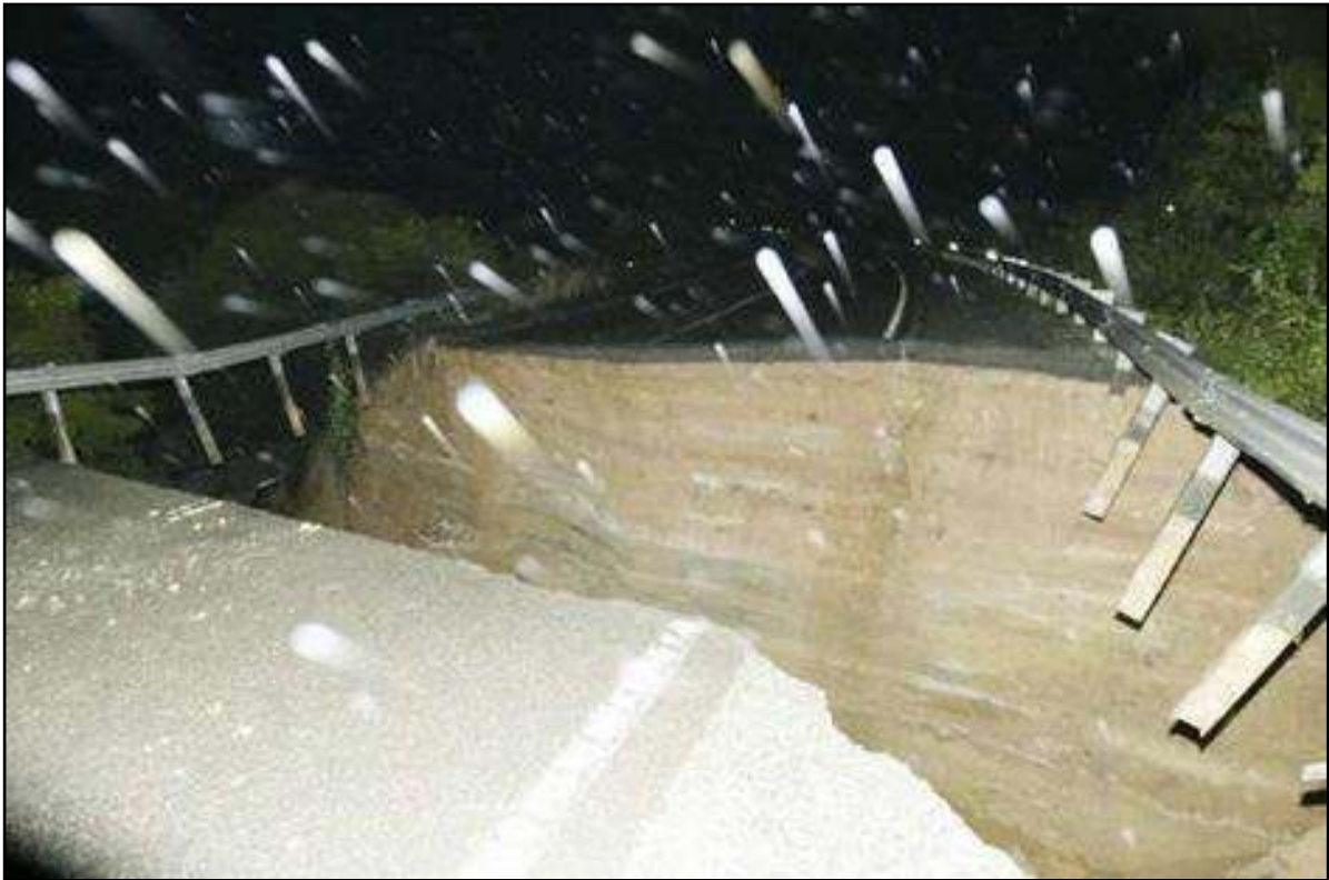
Figure 2: Old Pacific Highway road collapse at Somersby, NSW Central Coast, 8 th June 2007. Photo: Courtesy Daily Telegraph online news service.
