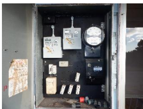
No termite barrier notice
