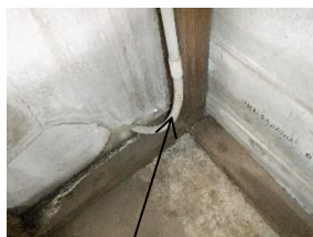
Decay to Garage frame
