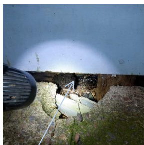
Laundry water leak
