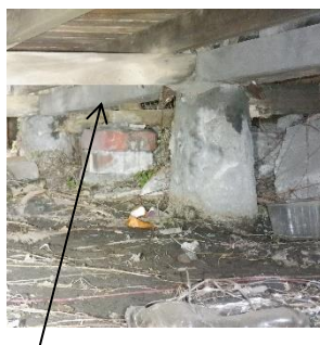
Missing termite shielding
