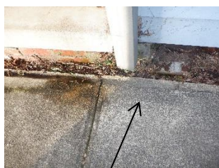
Downpipe discharge to ground
