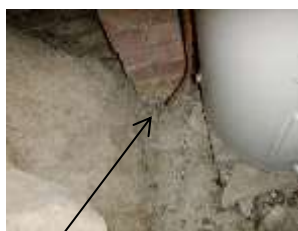
Heater drip pipe
