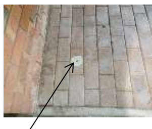
Termite monitoring station
