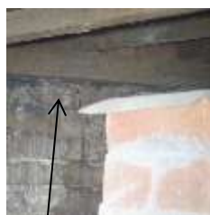
Corroded missing termite shields
