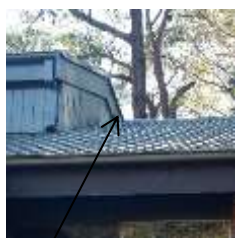
Decay to barge board
