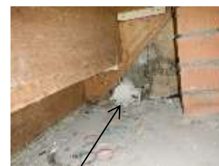
Previous water entry in lower level
