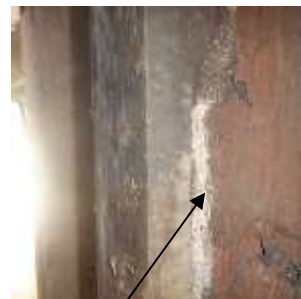
Active termite in shed (southwest corner)
