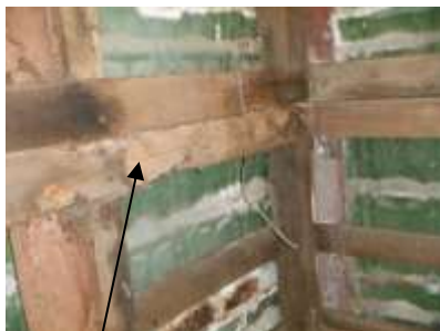
Termite workings in shed
