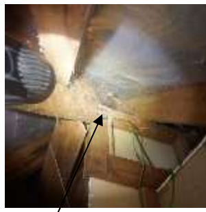
Termite working in roof frame
