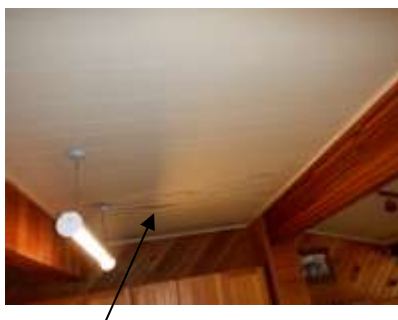
Previous roof leaks
