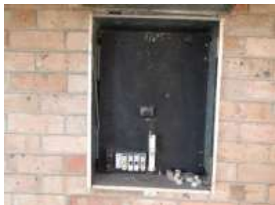
No termite barrier notice
